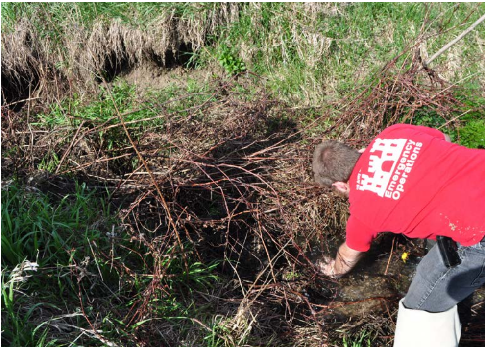
Anthony Heddlesten, environmental engineer, Environmental Engineer Section, Design Branch, Engineering and Construction Division, inspects a possible boil at Spring Lake Levee near Manito, Ill. Flood Area Engineers notified the Spring Lake Levee and Drainage District who arrived a short time later with plenty of sandbags to ring the boil. Photo by Felix Castro
