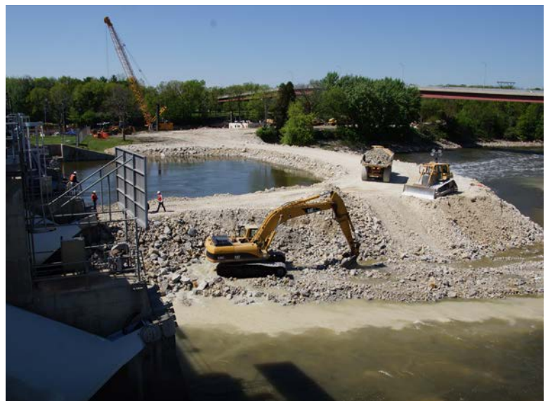
Rock Island District employees complete the rock dike just below Marseilles Dam during the four-foot pool draw down. Photo by Aaron Dunlop
