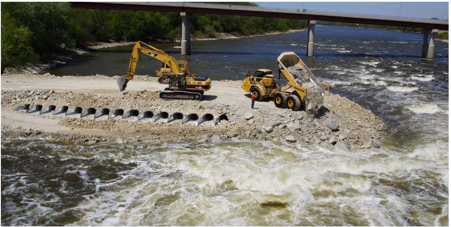
Rock Island District employees work to construct a rock dike just below Marseilles Dam. This dike helped reduce river flows and facilitate repairs to the dam. Photo by Aaron Dunlop
