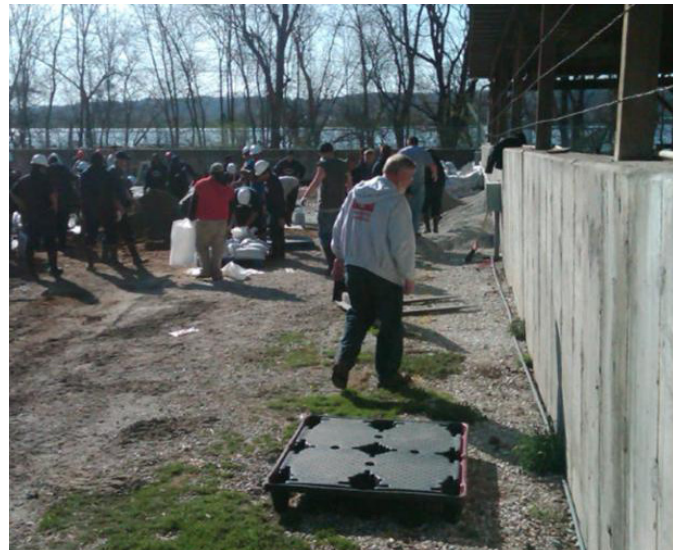
Larry Melaas checks along a concrete flood wall for seepage at Calihan Pork Processing in Peoria, Ill., April 22, In the background is a sandbagging operation to increase the level of protection at the plant.
