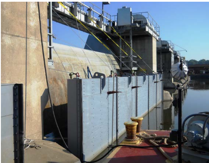
Bulkheads, fabricated by District employees, now block the flow of water through the Marseilles Dam.
