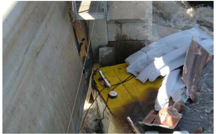
This photo shows damage to a concrete pier and the Tainter gate after alliding with Marseilles Dam. Photo by Aaron Dunlop
