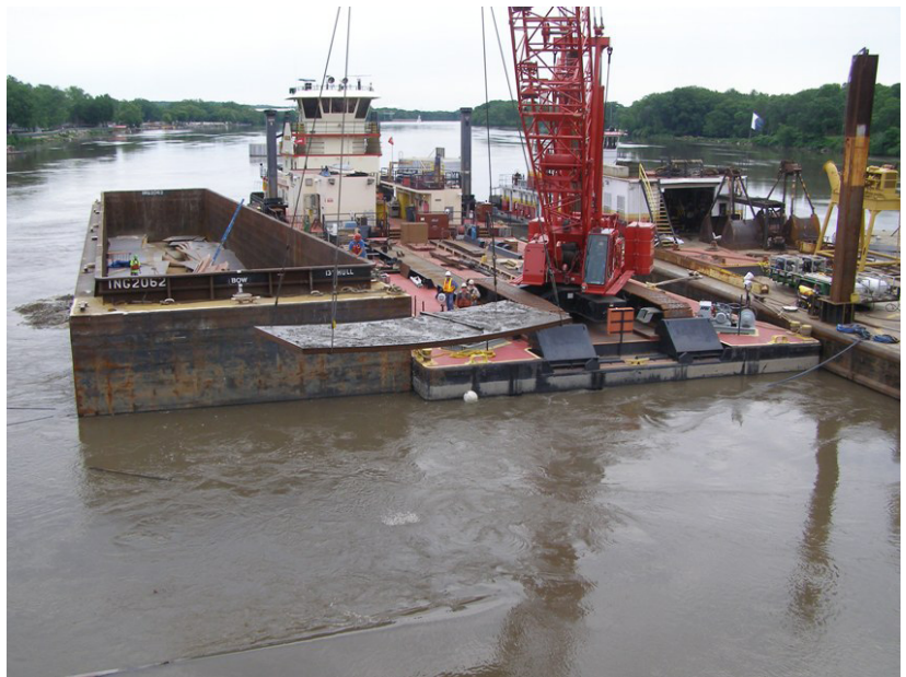
The District’s Manitowoc 777 assists the Unified Command in removing steel plates from one of the submerged barges at Marseilles Dam. Photo by Aaron Dunlop
