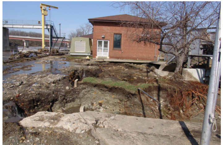
Significant erosion occurred on the north end of the dam near the Power House. Photo by Larry Rodriguez
