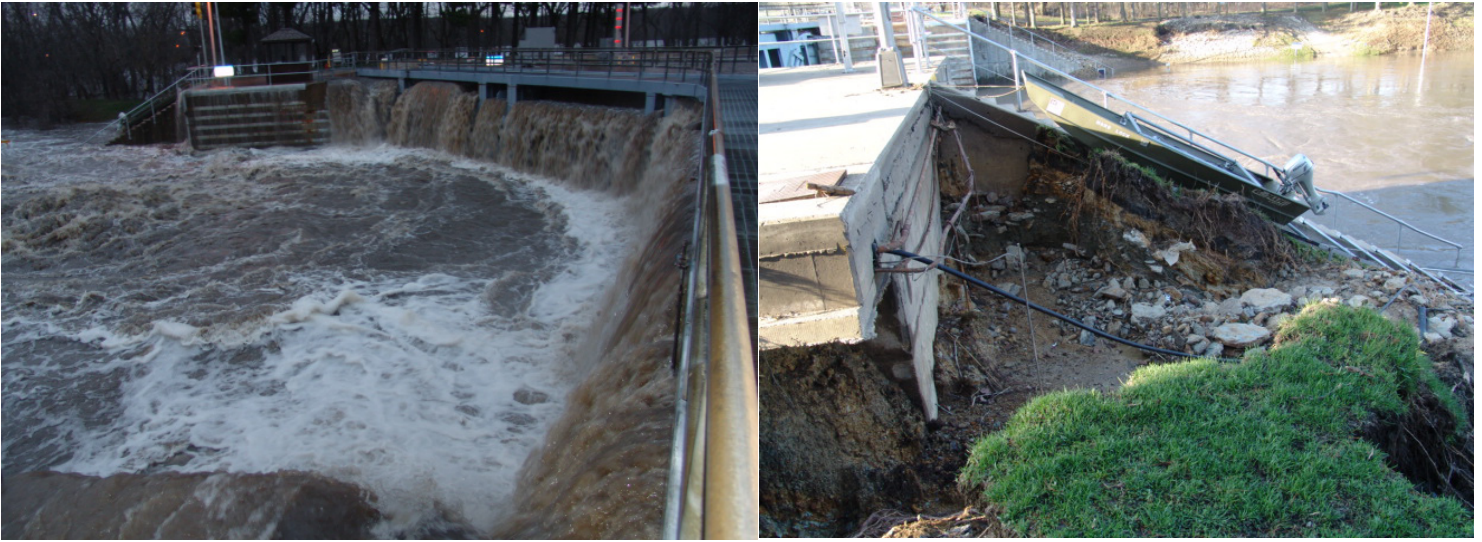
Significant damages occurred during the April flooding on the Illinois River. Left, water rushes over the lower miter gates at Marseilles Lock. Right, the water severely eroded the soil around the concrete wall and stairway just below the miter gate on the right descending side of the lock. Photos by Larry Rodriguez
