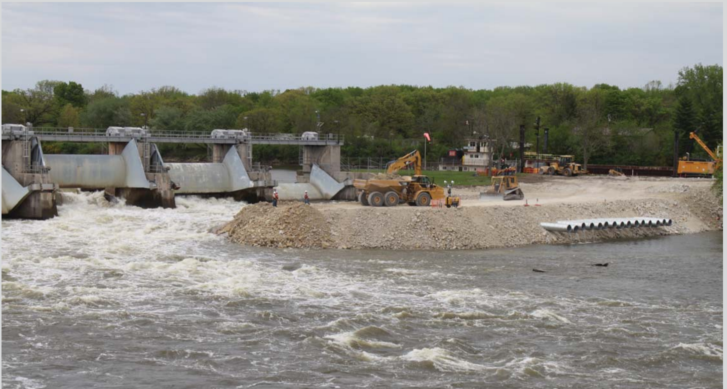
The rock dike shown here was part of the innovative plan developed by the Marseilles Dam Emergency Response Project Delivery Team following a nearly catastrophic incident that occurred in 2013. Designed in only a matter of days and built in just three weeks, this dike was a major part of the team’s plan. Photo by Allen Marshall
