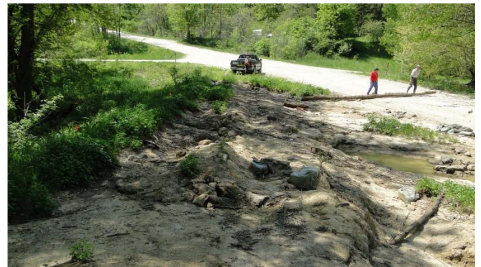
Photograph 171: Debris and Levee Damage (2013)
