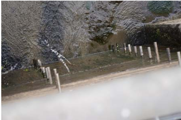
Photograph 24: Fox Pond Water Control Structure Stoplogs in Place (Mitvalsky, USACE 2016)
