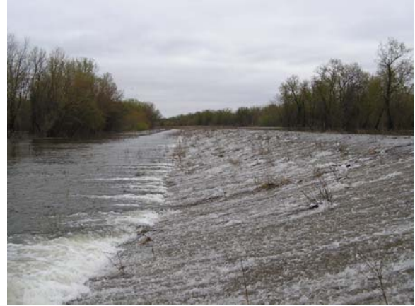
Photograph 86: Iowa River Spillway Overtopping (USACE 2011)
