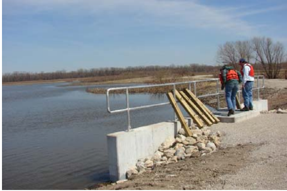
Photograph 23: Fox Pond Water Control Structure with Stoplogs Removed (Mitvalsky/USACE)
