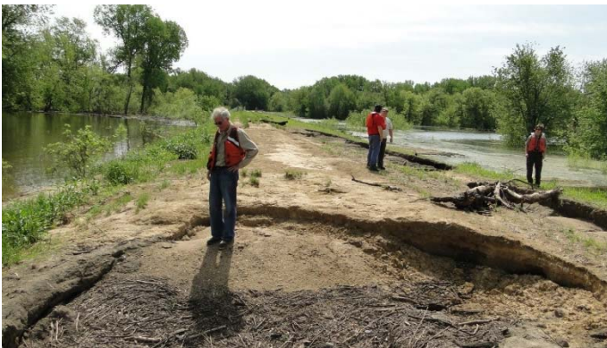
Photograph 168: 2013 Levee Damage Assessment (2013)
