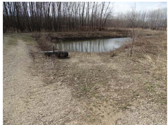
Photograph 9: Fields 4 and 5 Pump Pad (Mitvalsky, USACE 2017)
