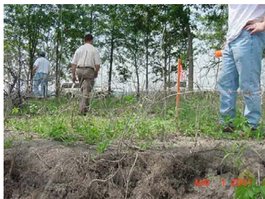
Photograph 197: 2001 Flood Damage Assessment (2001)
