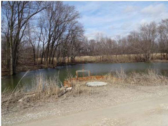
Photograph 18: Muscatine Slough Water Control Structure (Mitvalsky, USACE 2017)
