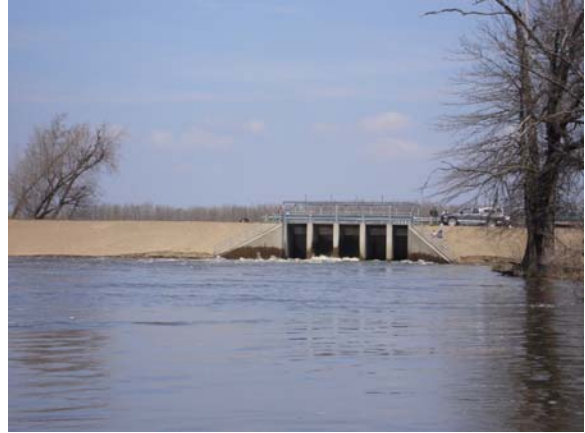
Photograph 74: Erosion at Outlet after Sand Enhancement and the 2008 Flood (USACE 2008)
