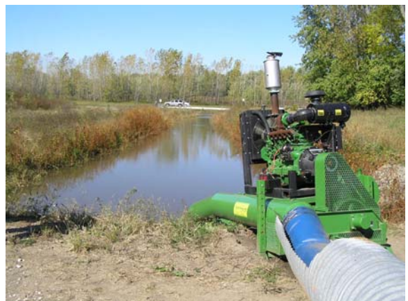
Photograph 15: Typical Temporary Pump, shown at Field 4 and 5 pump pad (Mitvalsky, USACE 2016)
