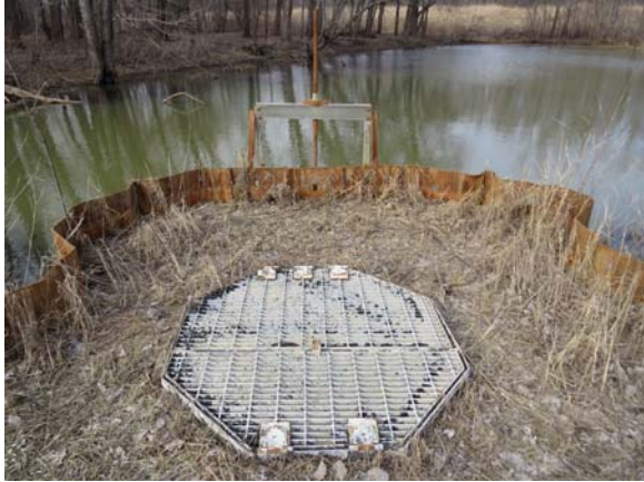
Photograph 17: Muscatine Slough Water Control Structure (Bolser, USFWS 2017)
