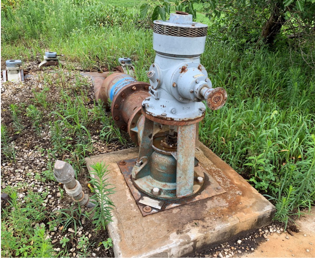
Figure 1. Existing Well Pump
