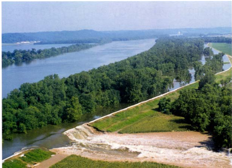
Figure 2.2: Levee Breach (North Central Division, 1994).
