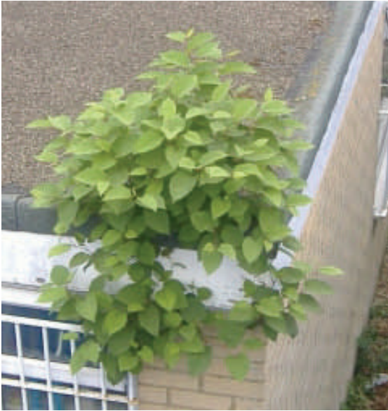
Japanese Knotweed growing in the gutter attached to a roof.
